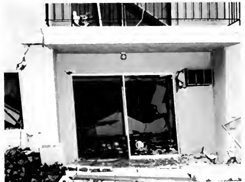
Photo 10. Portions of structures lacking adequate lateral strength sustained greater damage than those with adequate strength. Photo courtesy of the City of Los Angeles Department of Building and Safety.
